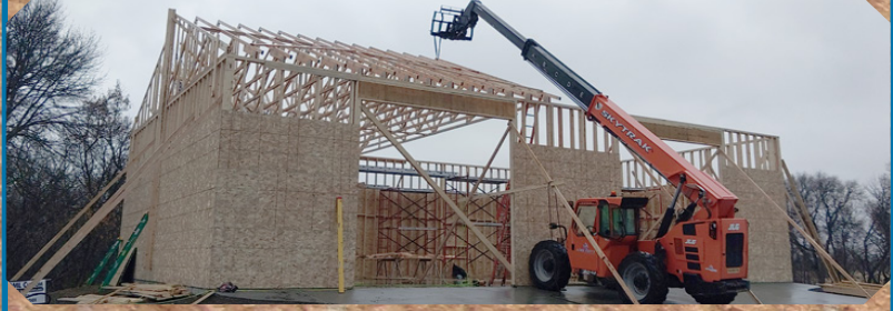
New Shop Build with CertainTeed asphalt shingles and LP Diamond Kote siding.
