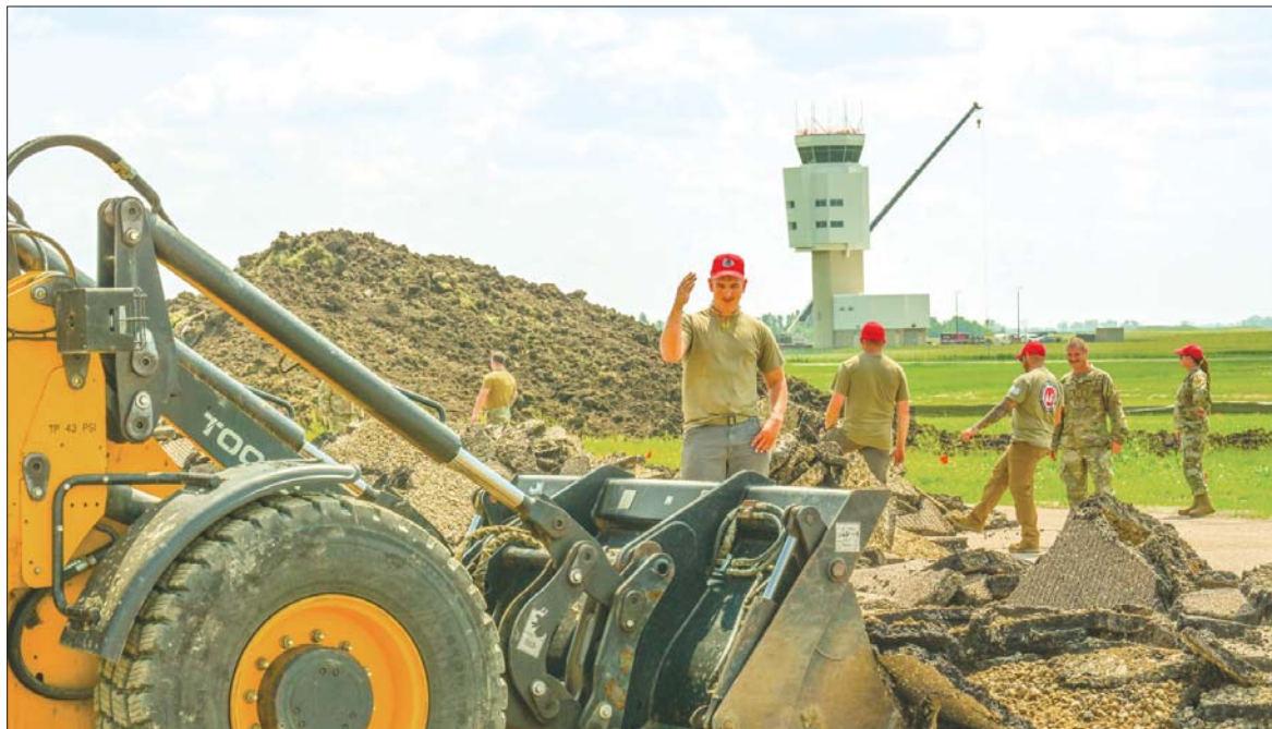
U.S. Air Force Senior Airman James Ludwig, 819th RED HORSE Squadron pavements and equipment journeyman, directs a plowman on the flightline at Minot Air Force Base, North Dakota, July 16, 2024. The RED HORSE Airmen traveled to Minot AFB to assist with removing and replacing damaged portions of the flightline as part of routine runway maintenance.
