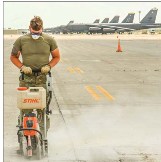
An Airman assigned to the 5th Civil Engineer Squadron removes damaged concrete on the flightline at Minot Air Force Base, North Dakota, July 16, 2024. The Airman used a concrete saw to separate, remove and replace damaged concrete as part of routine runway maintenance.
