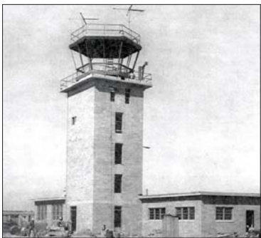
The original base control tower under construction in 1956. (Minot Daily News Photo)
