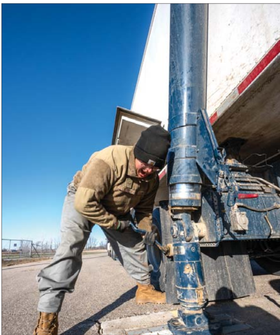
U.S. Air Force Airmen 1st Class Jonas Castillo, 91st Missile Maintenance Squadron mechanic, tears off the transporter erector from the missile site pad at Minot Air Force Base, North Dakota, Nov. 16, 2023. The Transporter Erector is used to lower the Minute Man III, into one of many missile silos around Minot AFB's area of responsibility.
