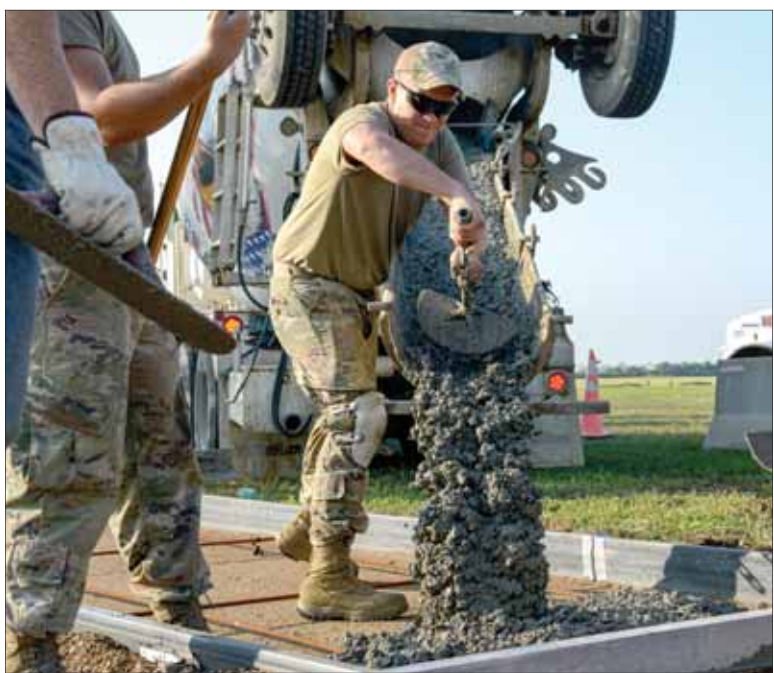
Air Force Staff Sgt. Tyler Cecil, 5th Civil Engineer Squadron pavements and construction equipment craftsman, pours concrete at Minot Air Force Base, North Dakota, July 20, 2023. The 5th Civil Engineer Squadron started construction on a sidewalk for a new airpark.
