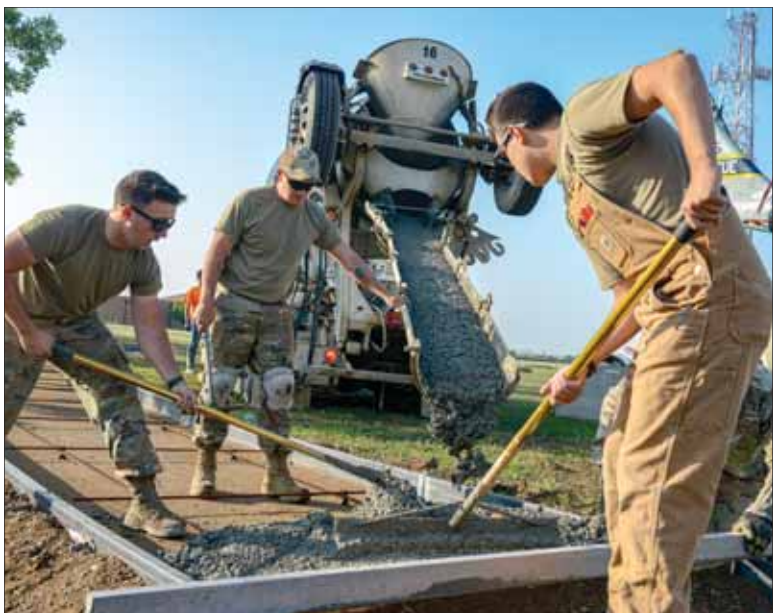
Airmen from the 5th Civil Engineer Squadron spread cement for a new sidewalk at Minot Air Force Base, North Dakota, July 20, 2023. This new path will allow families to be closer to static displays and enjoy Air Force history.
