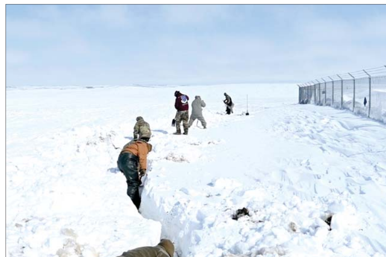
Airmen dig a trench April 26, 2022 at Minot Air Force Base, North Dakota. They shoveled over two feet of snow to prepare for the possible flooding from the melting snow.
