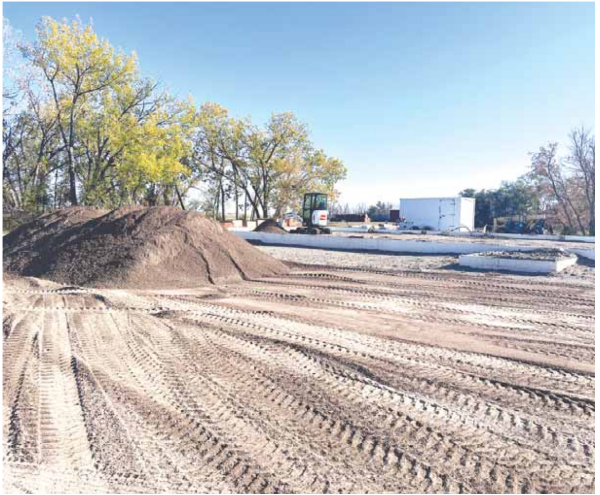
Construction continues at the site for the new Turtle Lake Ambulance hall.
