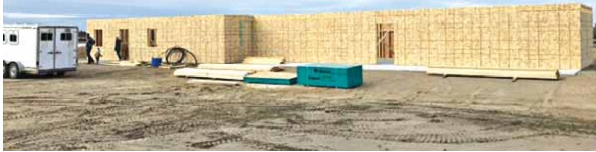
The partially constructed Sheridan Animal Hospital addition that will help serve the expanded service area of the facility in McClusky. The two buildings, a clinic and boarding kennel, will be located near the former livestock sales ring in east Harvey. Chris Tedford and Chris Arnold are general contractors for the project.
