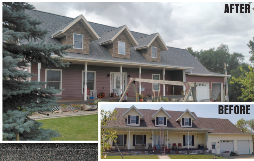
House remodeling project CertainTeed asphalt shingles, Mastic steel siding and Versetta Stone on dormers/garage
